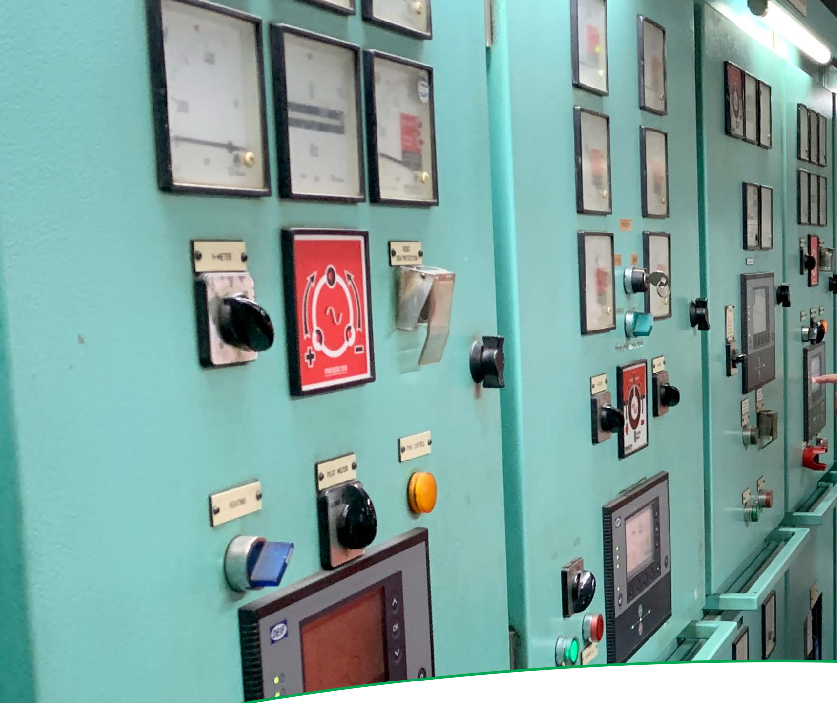
DEIF Senior Expert Engineer Didier Campeggio checks the status on a PPM 300 intelligent controller with the ship's Chief Engineer Nicolas Prebot in the technical room on board La Méridionale's Girolata.
